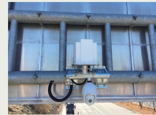
돌발상황검지시스템(AIDS) Automatic Incident Detection Systems
