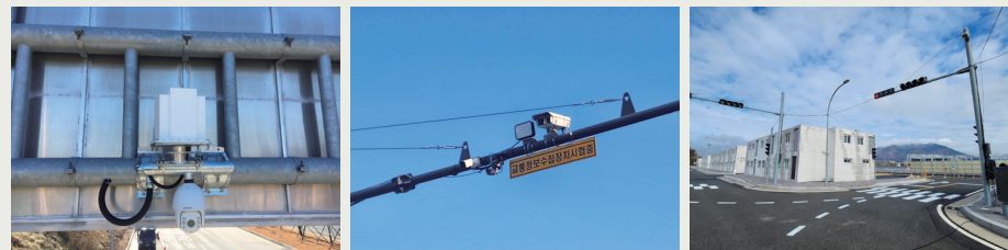
돌발상황검지시스템(AIDS) Automatic Incident Detection Systems | 차량검지기(VDS) Vehicle Detection System | 교통신호제어기(TSC) Traffic Signal Controller
