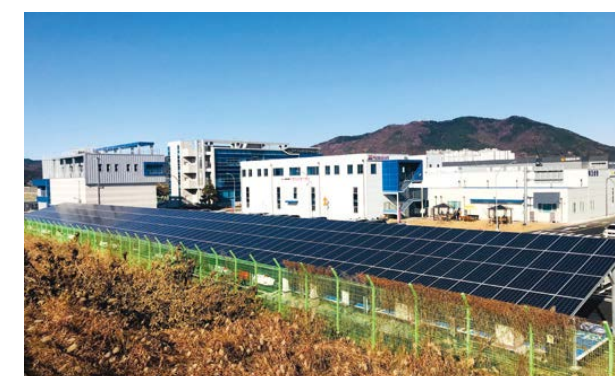
100kWh solar photovoltaic power station
